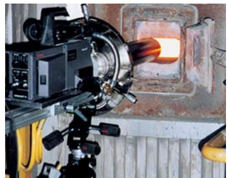
Special high temperature vortex tubes keep a boroscope lens cool while inserted into a 1200°F boiler porthole.
